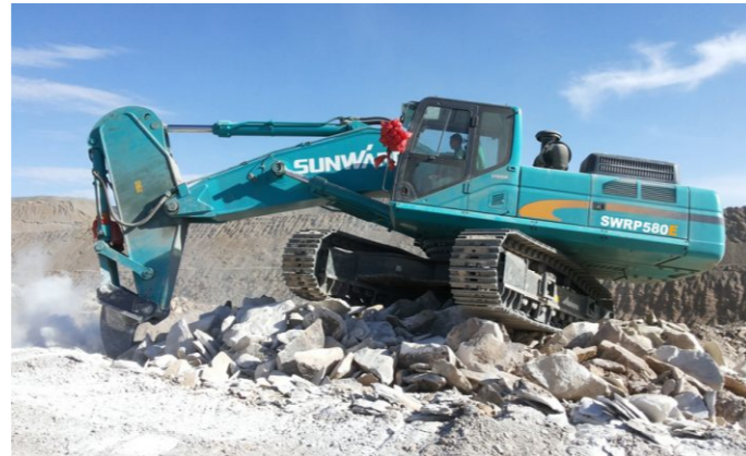
Hook-type Excavator Operating in a Limestone Ore Yard
